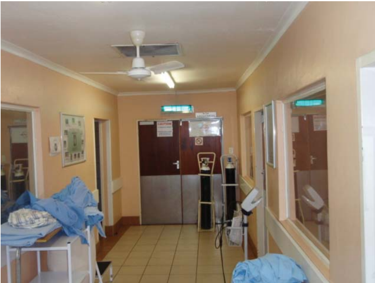
Figure 1: An upper-room germicidal UV fixture on the far wall, disinfecting the corridor between isolation rooms. Also shown in the foreground, a low-velocity ceiling fan assures good air mixing between the upper irradiated and lower occupied room.
